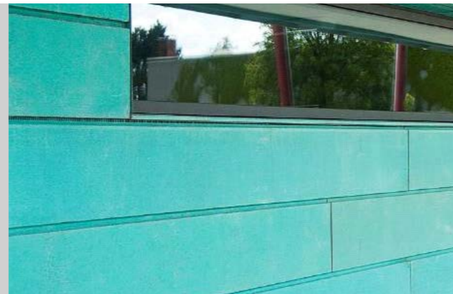
Special Education School in Dinkelscherben, Germany Architect: Frech & Mair Architekten BDA, Augsburg Photo: KME
